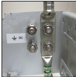
Fig. 11 – Grounding Cables Termination
